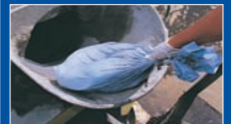
1 PREFORMULATED BAGS OF CCS PIGMENT CONCENTRATES ARE ADDED TO THE CONCRETE TRUCK AT THE PREDESIGNATED RATE OF ONE BAG PER CUBIC METRE
